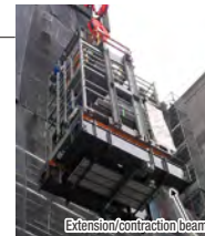
Machinery room unit
