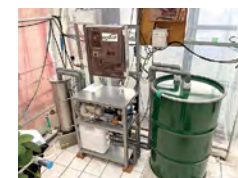
agleaf ® equipment installed
