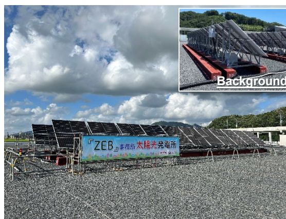
Photo 2: Solar power system at the field office
